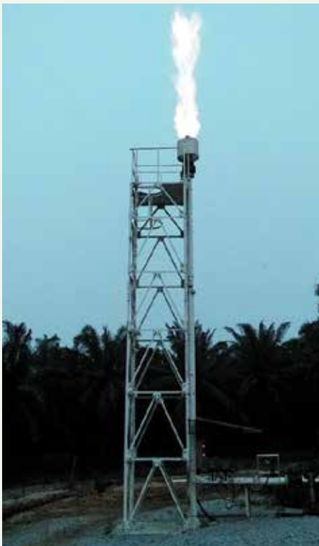
Telok Sengat Mill biogas plant – Flaring of excess biogas
